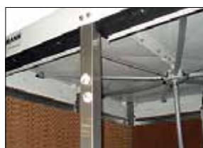
Water distribution system on the unit roof.
